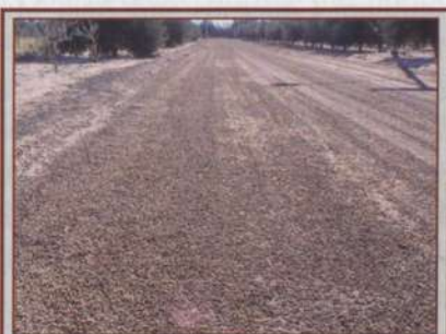
Fig. 12 Dirt road covered with olive stones
